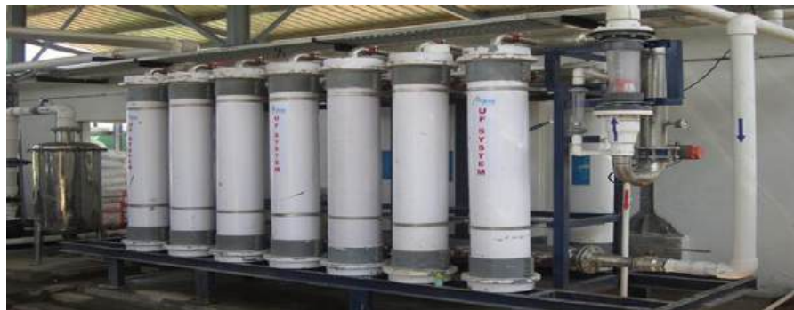
Case Study- Perungudi Sewage Treatment Plant
